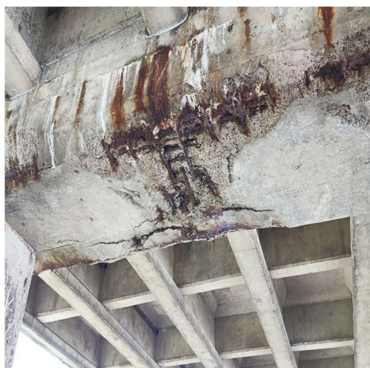
Figure 2. Severely exposed reinforcement and corrosion staining of a concrete bridge column cap.
