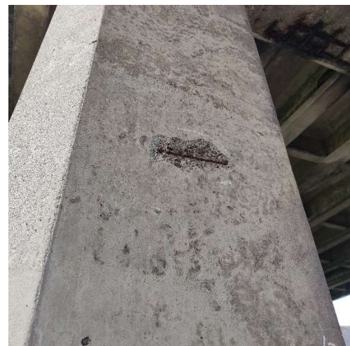
Figure 1. Minor exposed reinforcement and corrosion on concrete bridge column.
