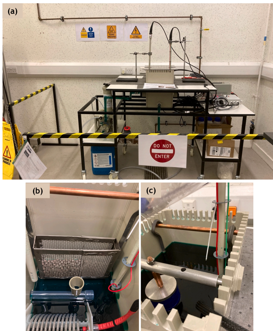
Fig. 6. (a) The complete prototype electroforming setup in the UoS workshop, (b) the anode basket filled with nickel pellets in the tank, (c) view of the filled tank with the titanium anode basket and a stainless-steel mandrel.
