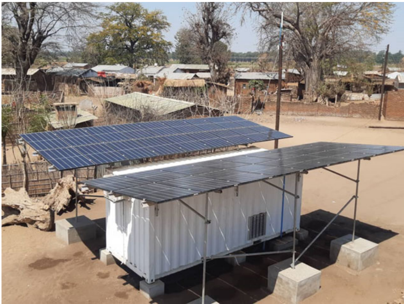
Fig. 5.6 12 kW solar micro-grid, Mthembanji, Malawi
