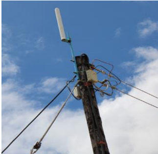
Smart meter antenna on a distribution pole (Mthembanji)
