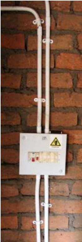
Customer premises wiring in conduit
