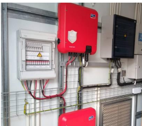
Inverters and controls within the shipping container (Mthembanji)
