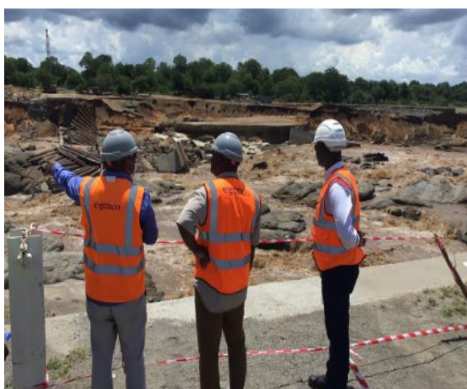
Damage to Kapichira hydro generation in 2021, Mthembanji remained functioning while most of the country experienced blackouts
