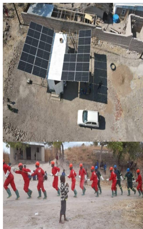
Kudembe generation under construction (top) and teamwork to run distribution cables (bottom)
