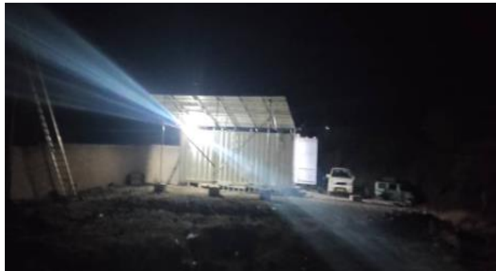
Security light at Kudembe generation hub
