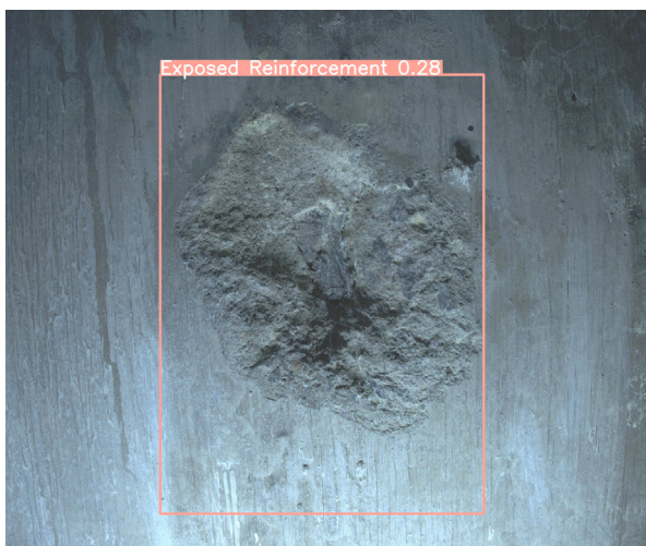
Fig. 22. YOLOv8 detection output of field trial spalling sample with low confidence exposed rebar detection.
