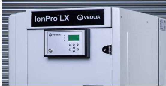
(a) Seawater desalination plant .
