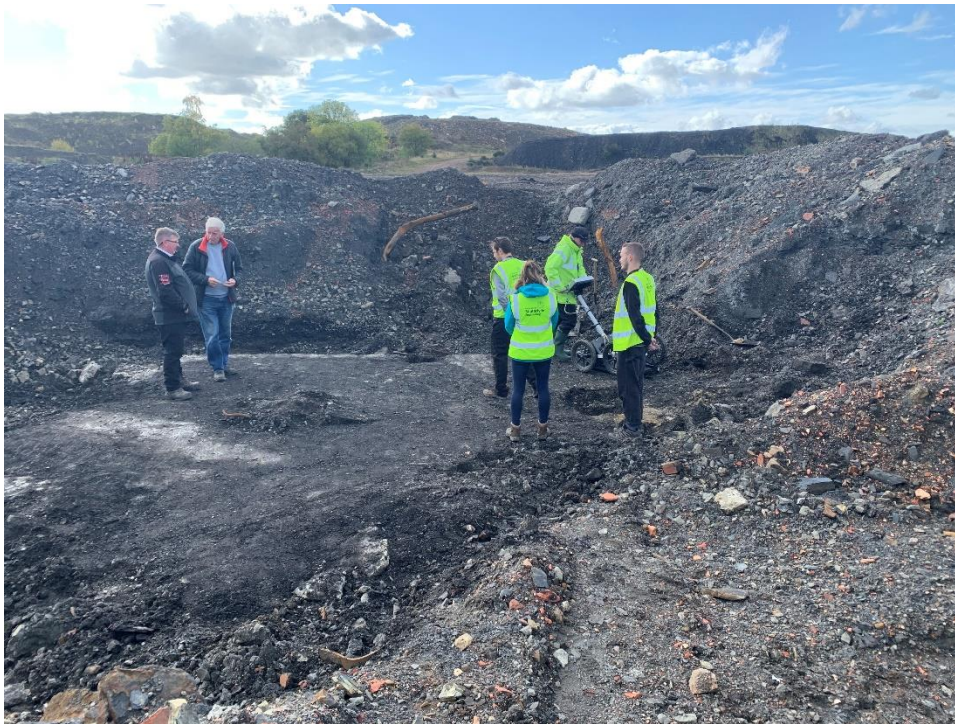
Figure 4: Photograph of the exposed concrete pad after excavation and GPR being set up for a survey.
