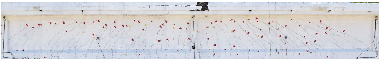
Fig. 15 Visible cracks on the middle portion of girder T4 opened during the loading phases P3 (amber triangles), P4 (red single triangles), and P5 (red double triangles) (colour figure online)
