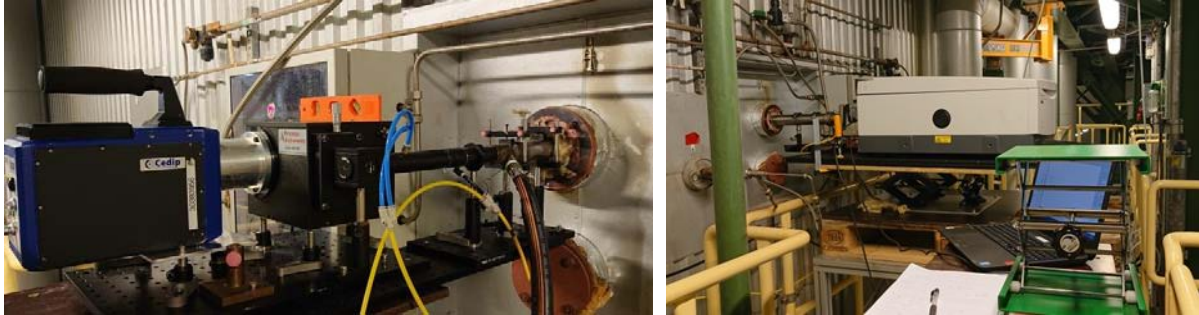
Figure 9. Parallel fast IR emission measurements with IR spectrometer and CEDIP IR camera (left panel: left boiler side) and FTIR spectrometer with sweeping probe (right panel: right boiler side). Both systems are viewing the same axis.
