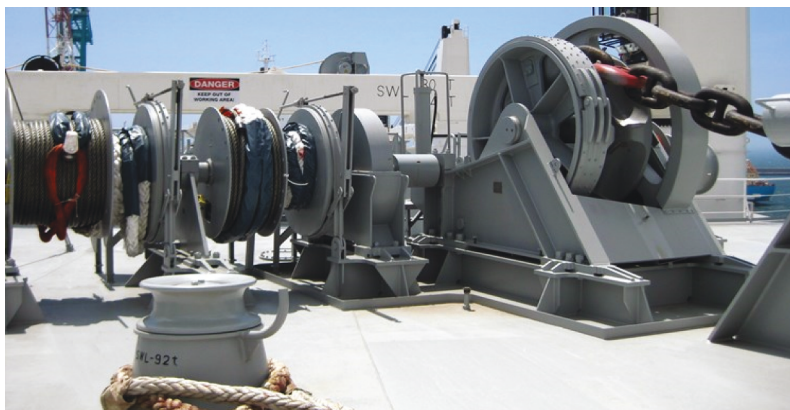
Figure 9. Mooring winch (Aicrane, 2022).
