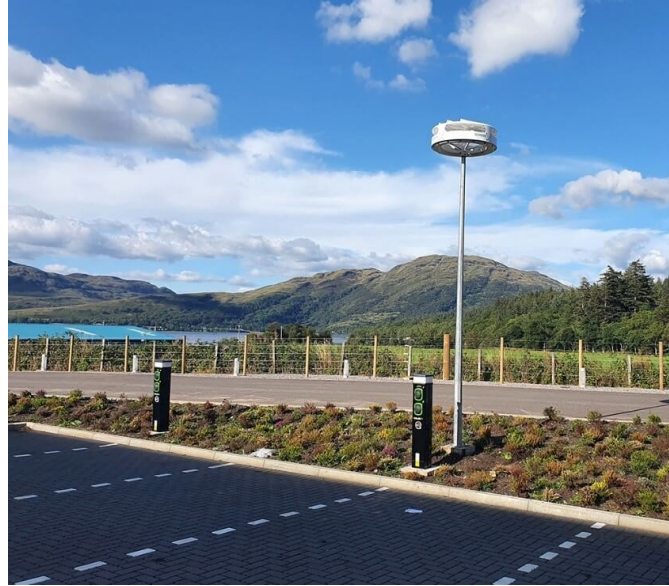
Fig. 2: Example of Autonomous-IoT smart streetlight next to an EV charger.
