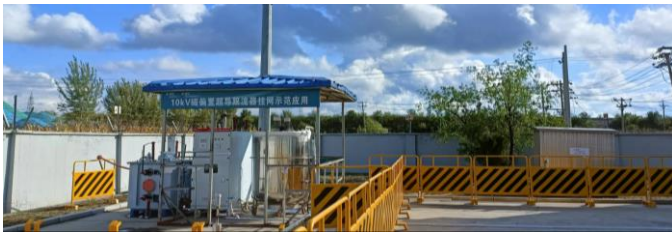
Fig. 8. The photo of site of grid-connected test.
