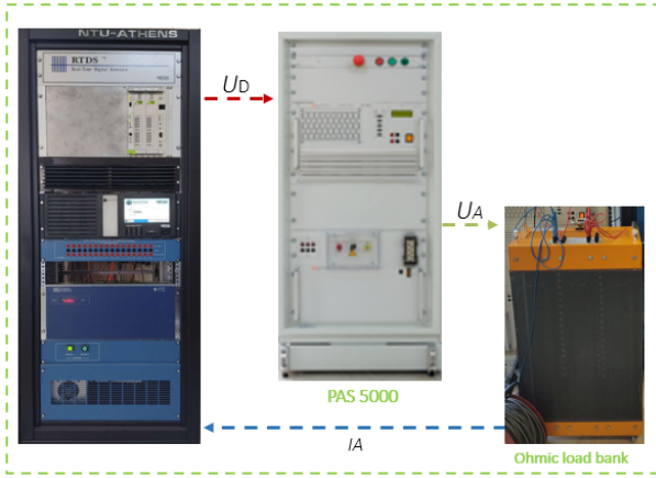
FIGURE 12. Experimental setup of the implemented PHIL simulation system with applied V-ITM interface.
