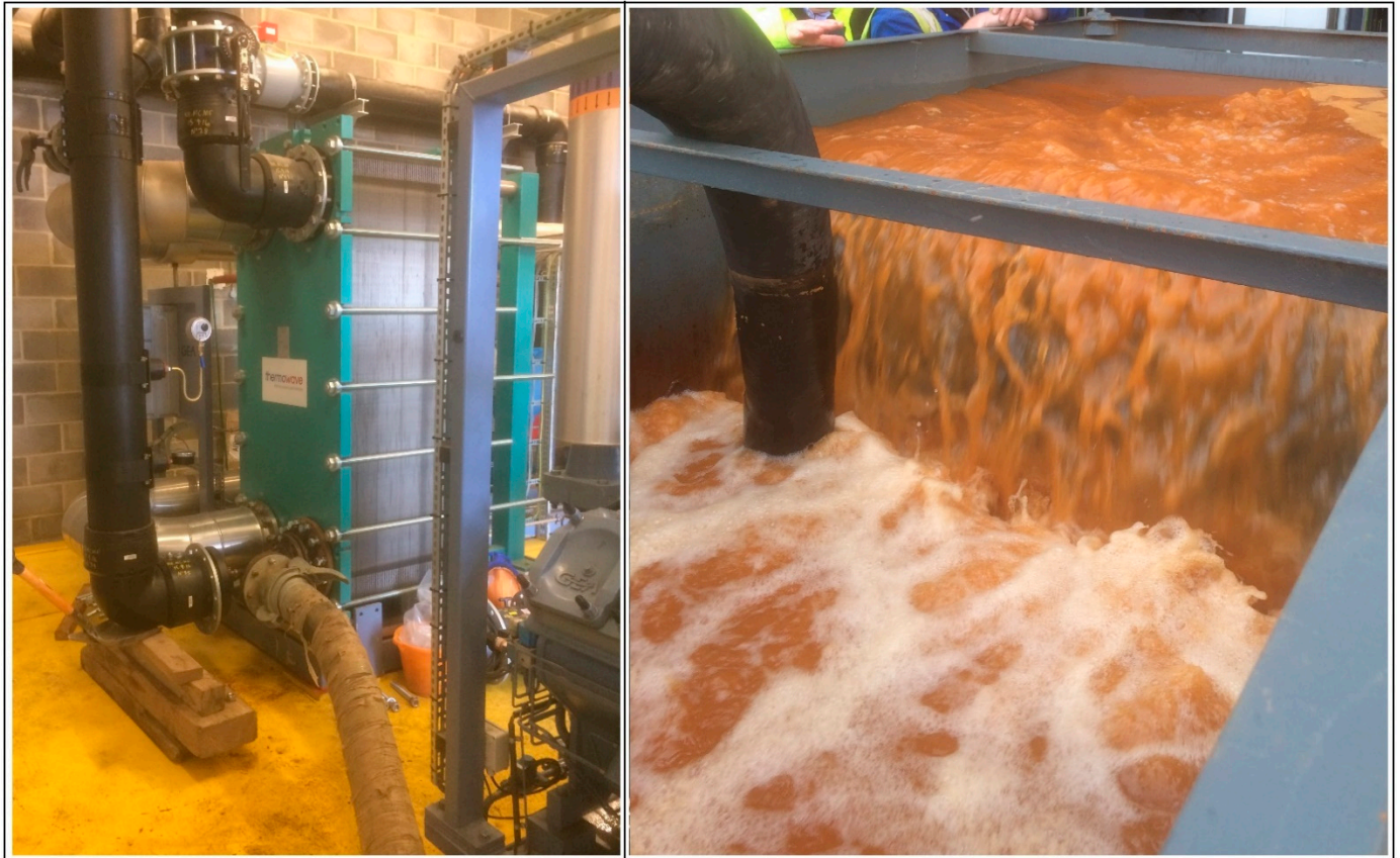
Figure 4. Periodic recirculation of citric acid solution through the plate heat exchanger at Abbotsford Road, Gateshead, UK ( left ), to remove accumulated ochre (which can be seen in the recirculation tank, ( right )). Reprinted with permission from ref. [70]. Copyright 2019 David Banks.
