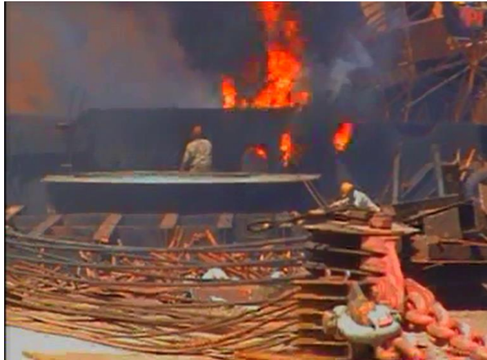
Figure 1: Fire caused by burning the residues on blocks
