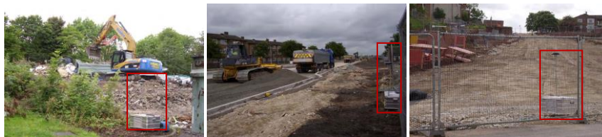
Fig. 1: Positions of dust analyzers. Left: demolition activity. Middle: earthwork. Right: site entrance. Pictures from HSE (HSE, 2011).
