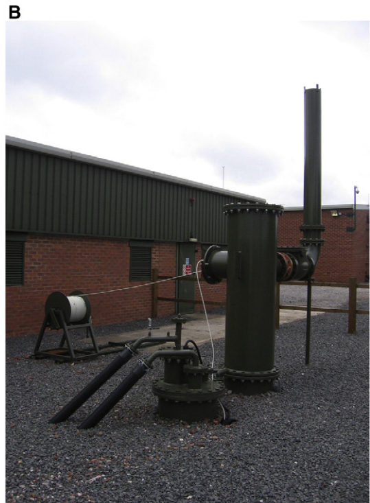
Fig. 3. Upper- the headworks of Markham No. 3 Shaft, showing methane venting and the (angled) pumping and return mains of the 'standing column' heat pump system. Lower- shell and tube heat exchangers in the heat pump plant room. Photos by D. Banks.
