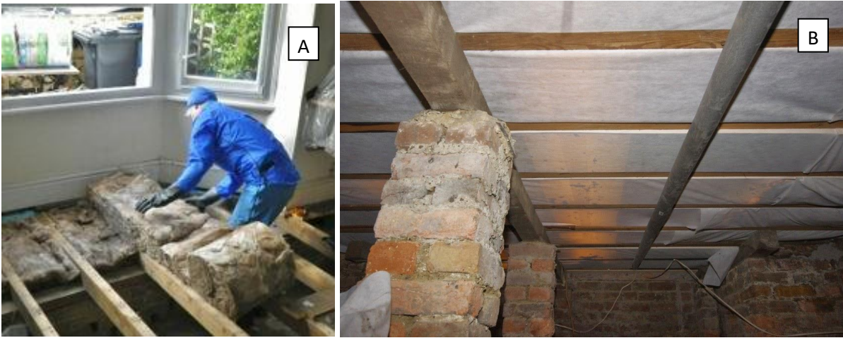
Figure 2.3: Underfloor insulation can be applied to suspended floors from above after removing floorboards (A) or from below (B). (Bragg, 2012; MacKay, 2015).
