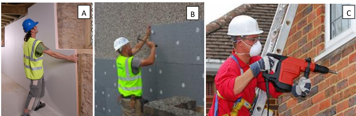
Figure 2.2: Forms of wall insulation: A internal; B external, C cavity fill. (Source: NIA, 2020).
