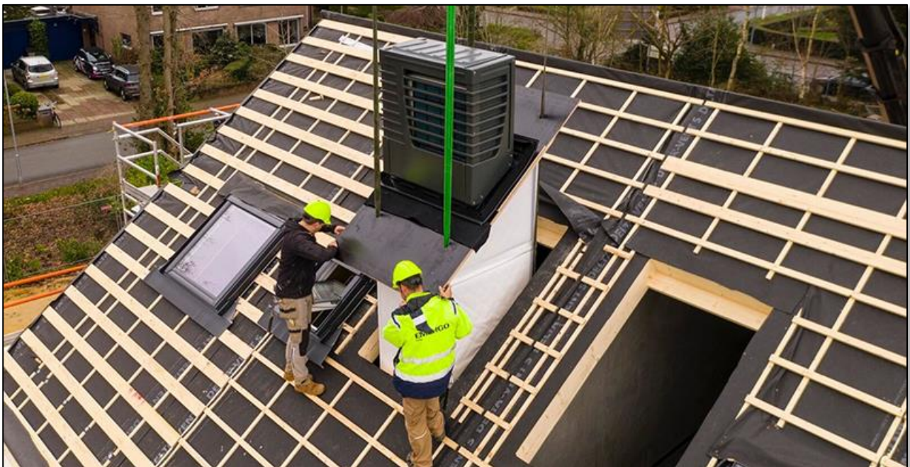
Figure 3.3: A plug and play energy unit combining heat pump and battery storage being lowered into place in social housing in the Netherlands. (Source: Energiesprong, 2020).
