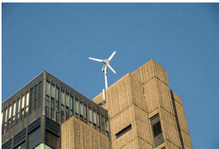
Fig. 6. Roof mounted turbine
