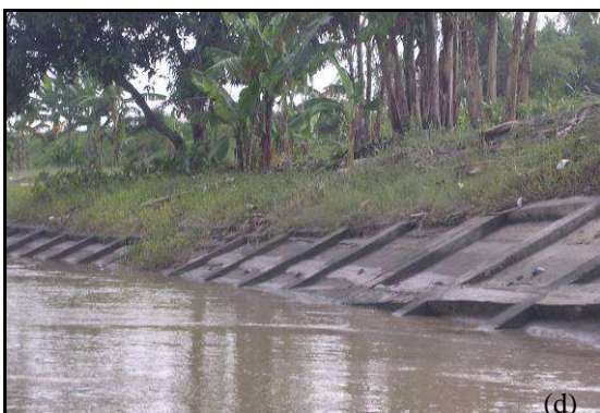
Fig. 2. Failures along the Bengawan Solo Embankments: (a) erosion of natural embankments; (b) shallow failure of man-made embankment; (c) global failure of gabion reinforced embankments; (d) differential settlement under concrete protection slabs.
