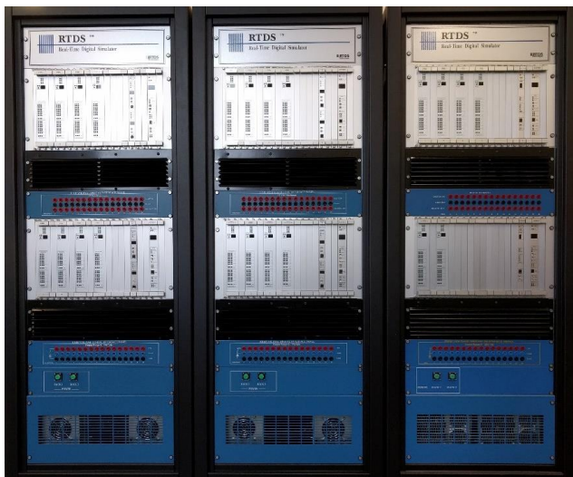
Figure 1 RTDS Hardware (cubicles)
