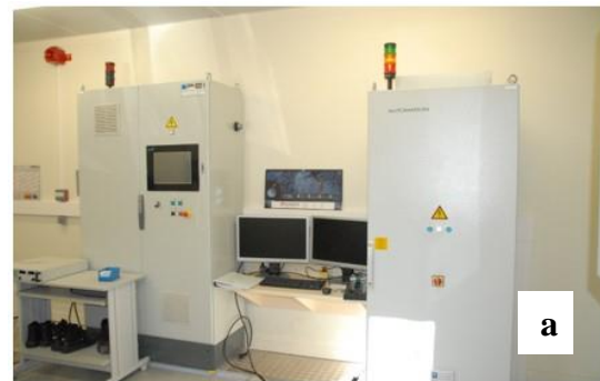
Fig. 9.a. Li-ion batteries measurement system
