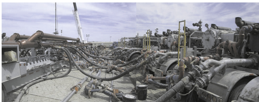
Fig. 5. Photograph of the site showing high and low pressure pipework connecting positive displacement pumps (right) to a manifold trailer (left) on hydraulic fracturing site. Photograph was obtained from south Texas.
