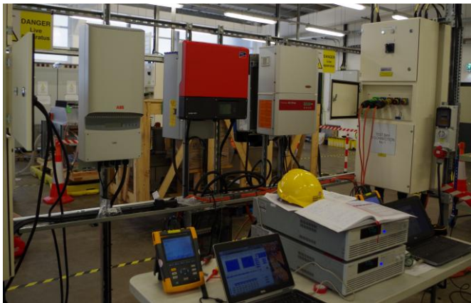
Figure 7 Inverter testing setup at the PNDC
