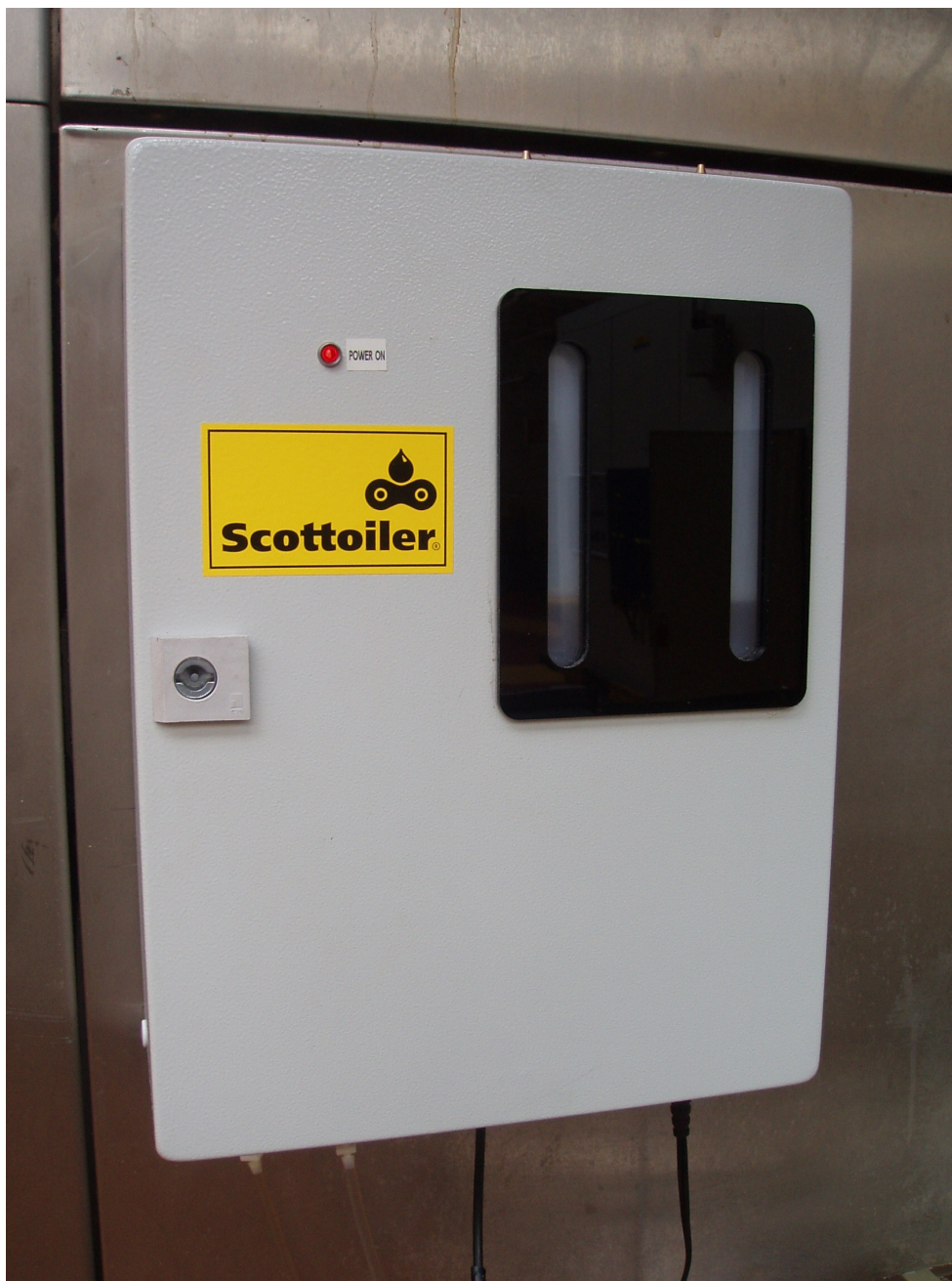
Prototype II in installed position
