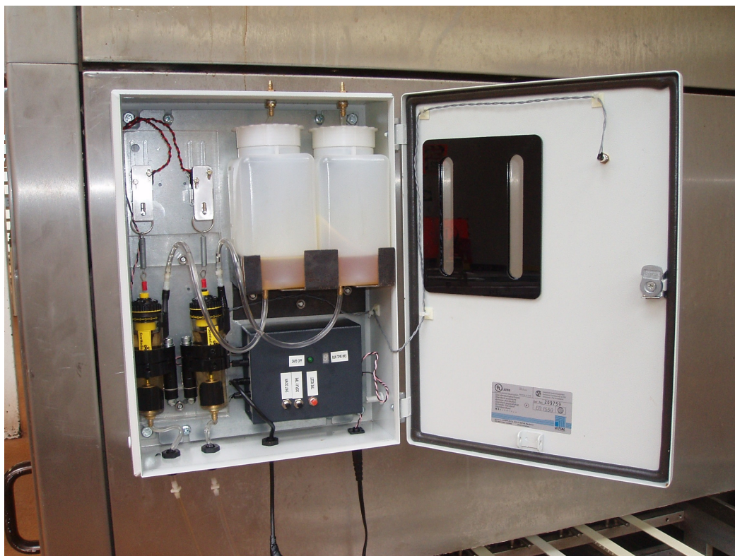
Prototype II in installed position
